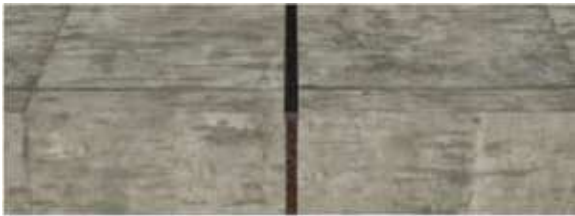
Continuous expansion joints
